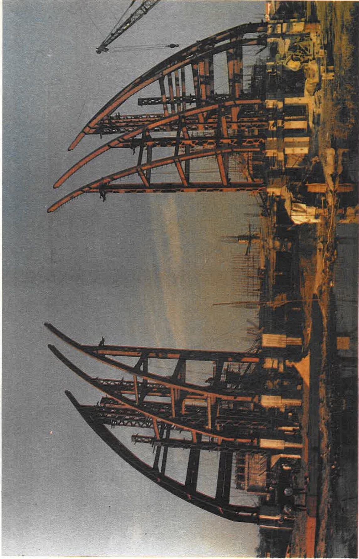
Work in full swing at the Science City Project of National Council of Science Museums at Calcutta
